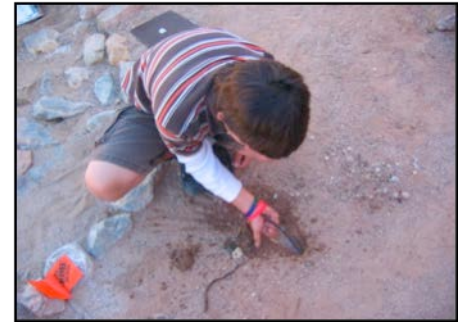
Student investigating and flagging broken drip tubing.
